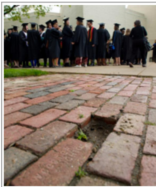
Campus Grounds crew was kept very busy replacing the Wooster bricks that were "removed" from Taylor Hall sidewalk this past spring.
